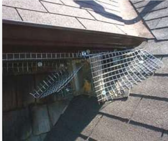
Exclusionary mesh and a one-way door installed around a raccoon entry under the overhang where the roof of a gable meets the main roof – a favored spot for wildlife entry into attics.
