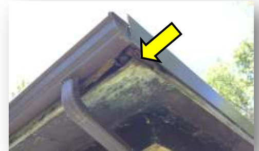
Water damaged wood caused by clogged gutters. Such damage creates openings for wildlife into your home
