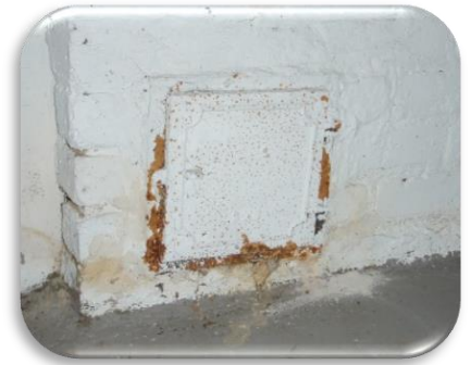
A typical clean-out door at the bottom of a chimney in the basement. These usually measure about 12" x 12". This one doesn't look like it has been opened in many years and is rusting around the edges.
