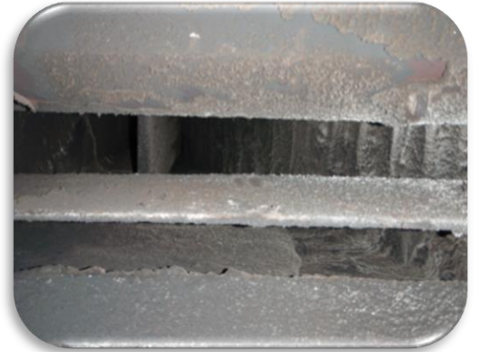
Though fireplace damper styles vary, this is what a typical damper looks like in the "open" position. This view is looking straight up from inside the fireplace.
